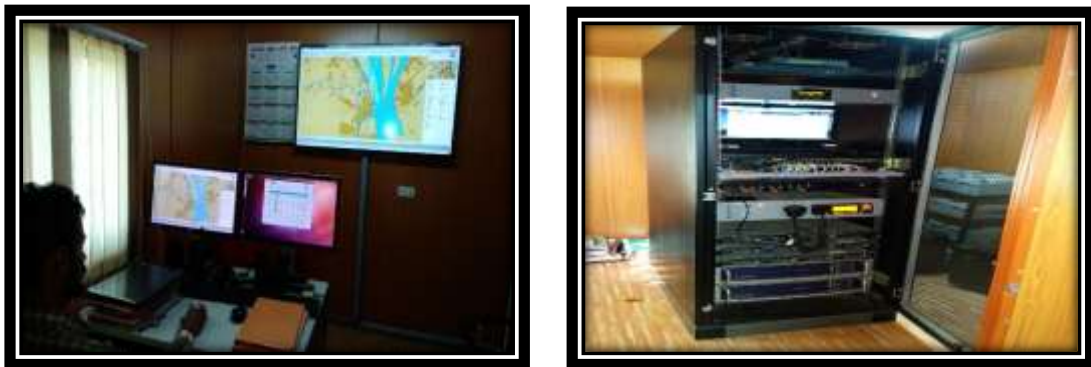
(Fig No.23. View of RIS+DGPS Equipment & real-time Metrological Monitoring of National Waterway 1) 20
