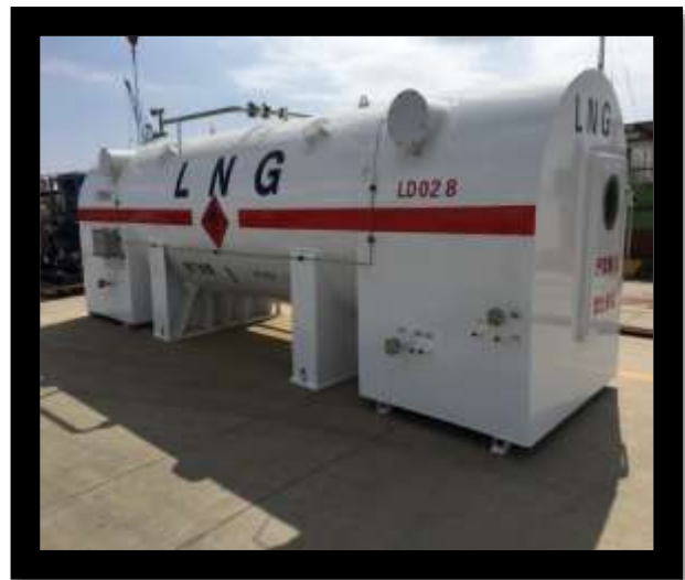
(Fig No.27. View of Fuel Bunkering Station along NW-1)
