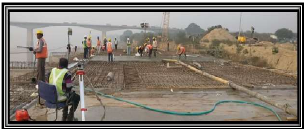
(Fig. No. 197. Construction of Varanasi MMT on going by M/s AFCONS Ltd)
