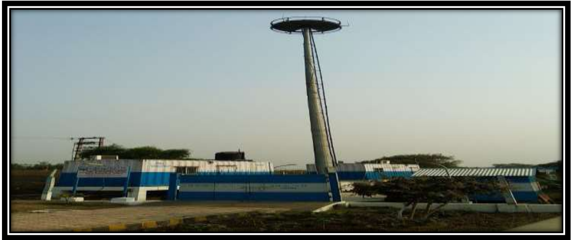
(Fig No.22. View of DGPS & River Information Stations Installed along NW-1)
