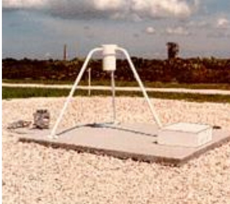
Fig 3.2 Electric Field Mill Installation at Kennedy Space Research (Florida)
