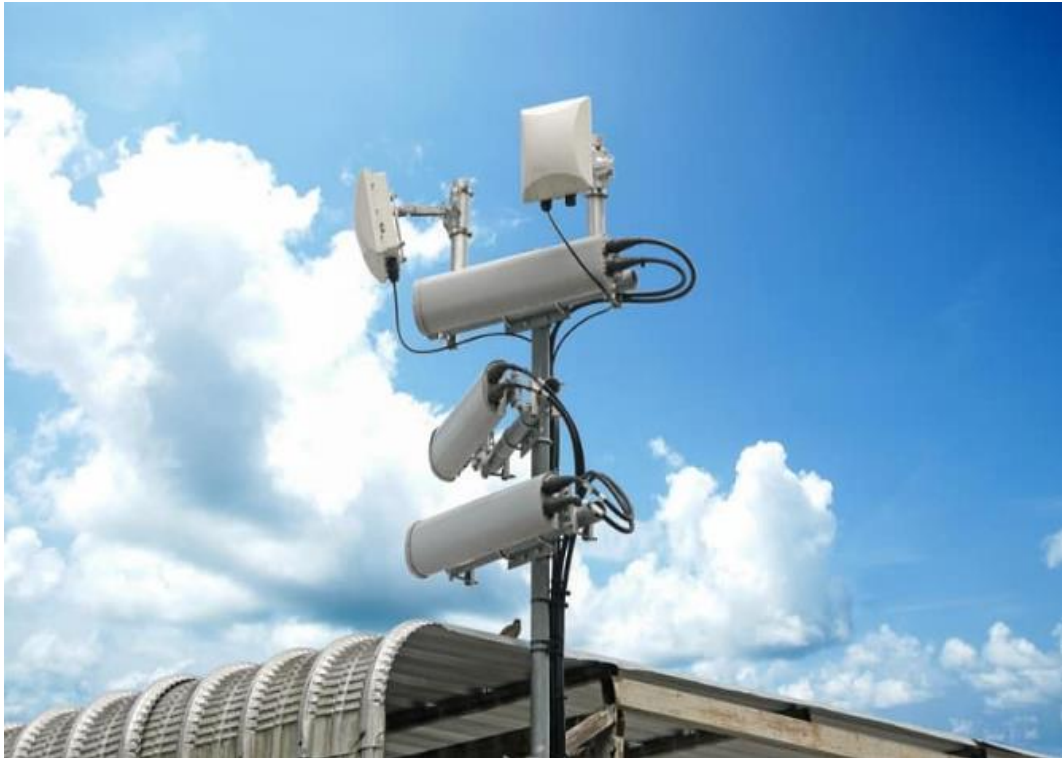
Figure 1.12:Advanced wifi antenna for long distance
